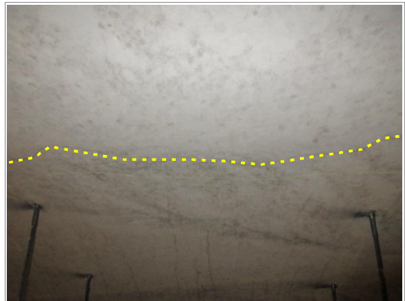
Span61 천단부 균열(cw=0.3mm/9.0m)
